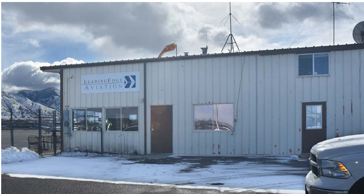
Figure 18: This is the exterior appearance of the Leading Edge FBO at LCCA. It is dreary and industrial. This deficiency cannot be blamed on Leading Edge; the airport owns this building and leases it to the FBO.
