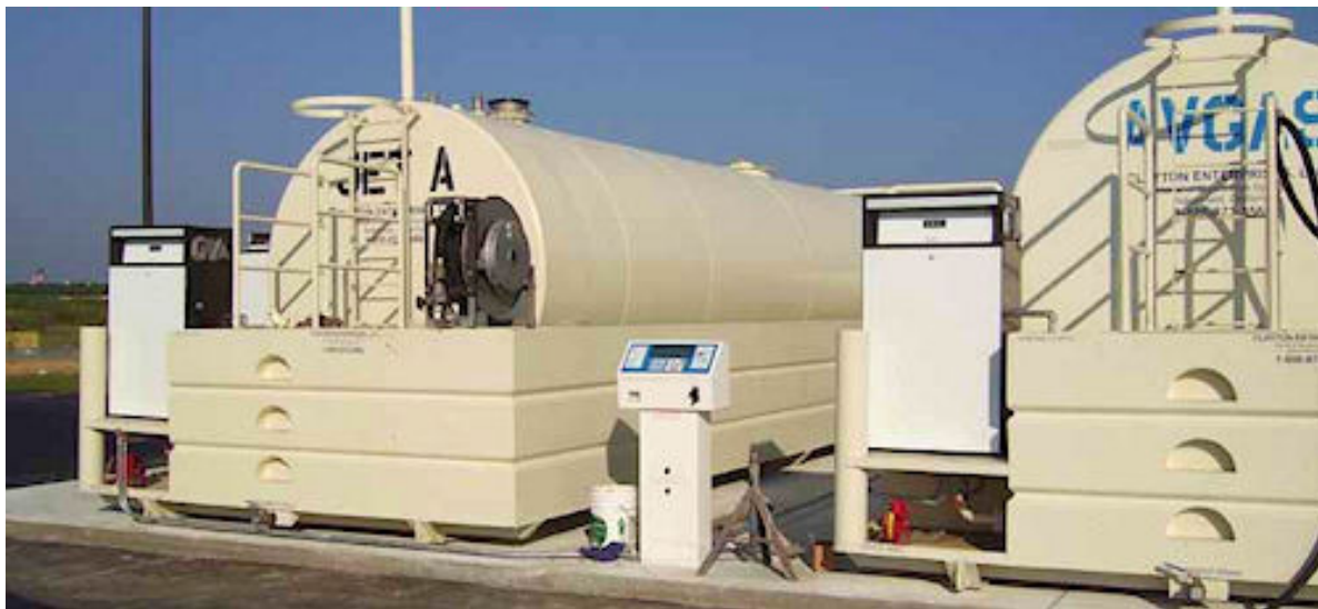
Figure 22: This illustrates a typical "self-serve" refueling system. It has two tanks, one for Jet-A and one for 100LL. It processes payments using a credit card reader.
