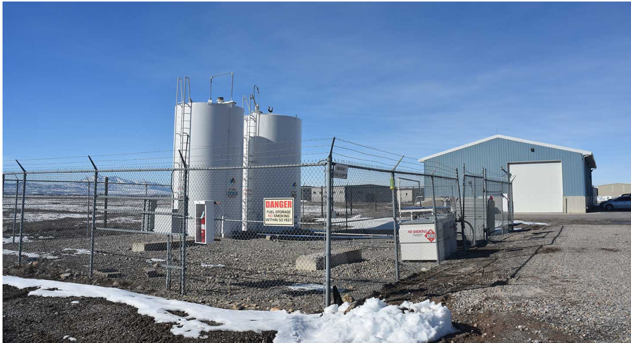
Figure 14: The LCCA fuel farm was installed in 1969. It is too small and functionally obsolete. It does not comply with modern Part 139 fuel farm standards.
